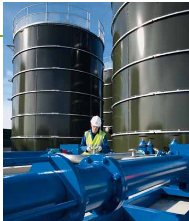
Water treatment facilities for Anglian Water, U.K.
