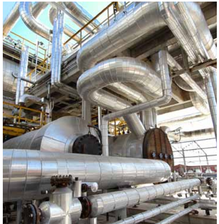
Petrobras Sulfur Recovery Unit, São Paulo, Brazil.
