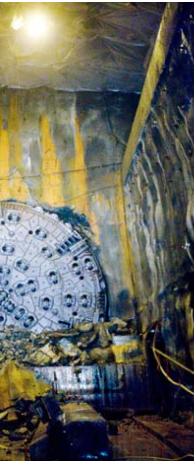
In August, a milestone breakthrough was achieved at the Hallandsås (Hallandsås Ridge) rail-tunneling project in southern Sweden. The tunnel-boring machine, named Åsa, completed the first of the two 5.5-kilometer pipes. The final breakthrough is planned for 2015.
