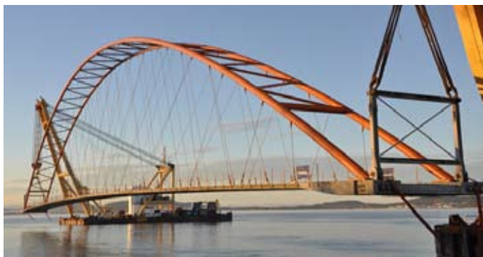
The 285 m (935 ft.) long bridge over Brandangersundet to Sandøyna, Norway was fabricated and installed by Skanska.
